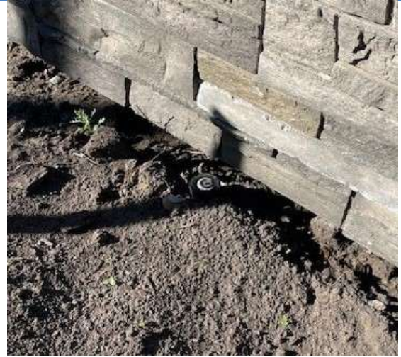
Irrigation Spray Head
