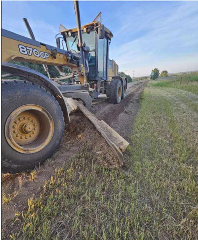
Shoulder pull on Range Road 234
