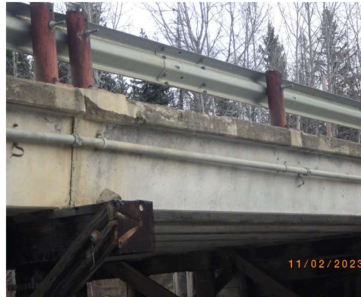
Concrete spalling from girder
