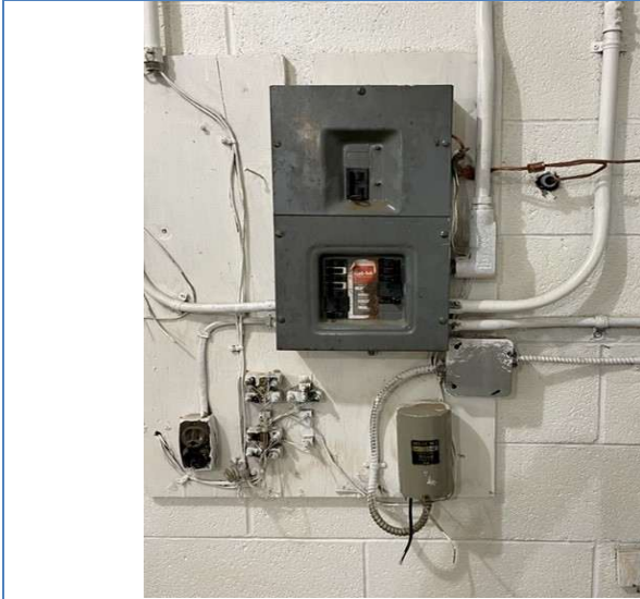
New Sarepta Shop - Electrical Panel
