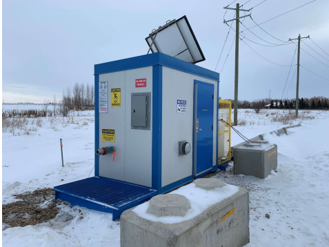
Bulk water fill station
