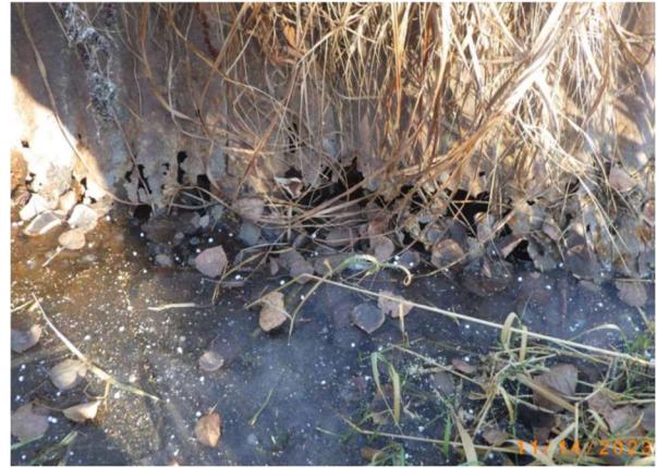
Extensive perforations in culvert floor
