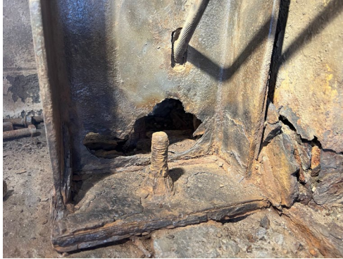
Corroded steel column
